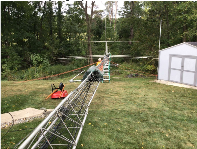
10 days later, Tower with new antennas, coax and cameras ready to go up.
